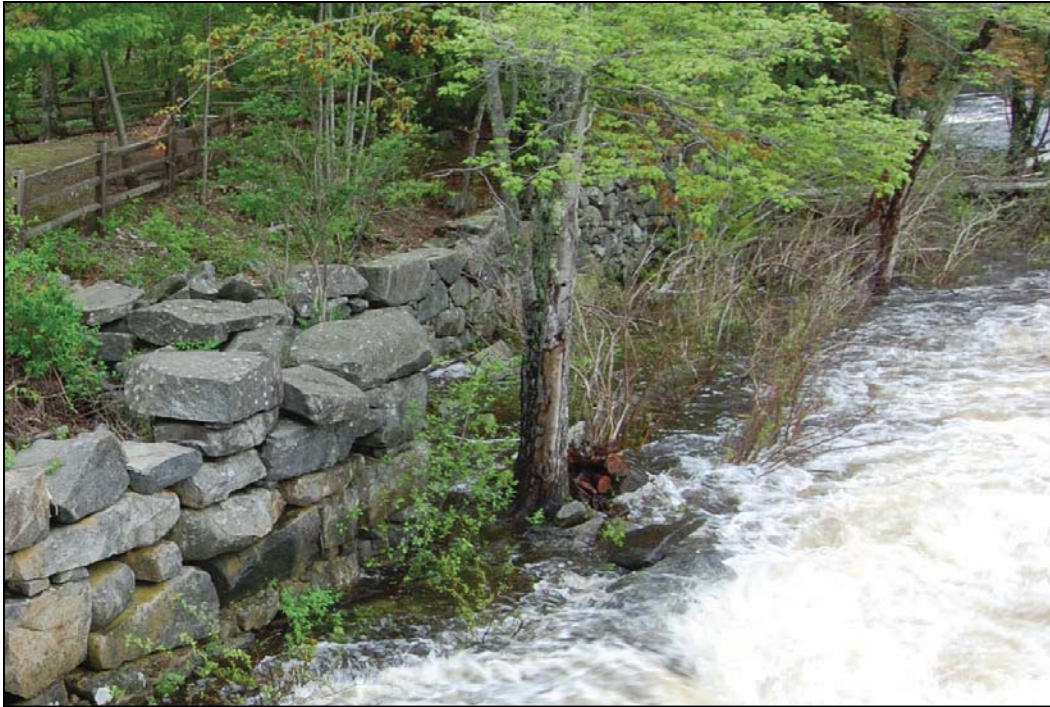
Photograph 15. Structure 10 – Grist/Flour Mill Foundation, west foundation wall downstream (south) of Sawmill Foundation.
