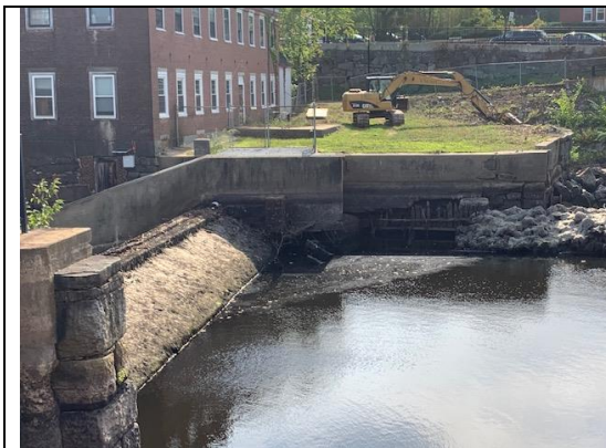
South side: Pre-construction drawdown complete. Damage to the wall is visible between water and upper concrete. Sept. 7, 2020
