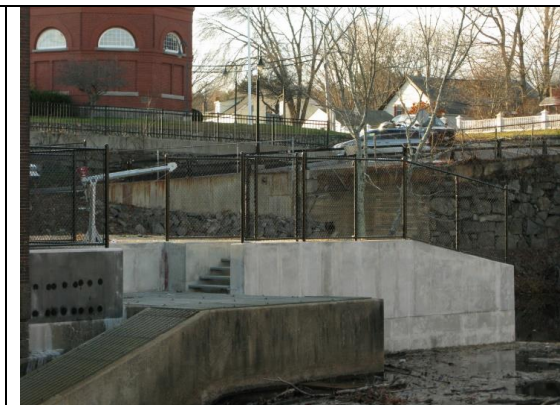
The overall height of the reinforced south wall is about 4 feet higher than it was. New stairs leading to the fish ladder holding tank are visible. New fencing has been installed. Nov. 18, 2020
